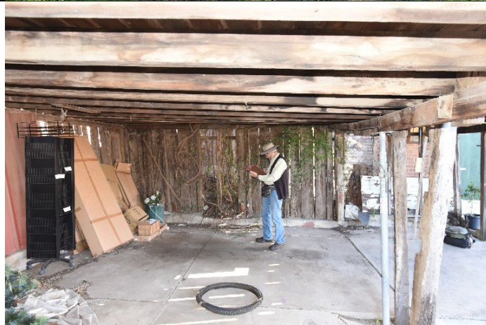
Caption: Town barn at 117 George Street, Windsor (interior) Photographer: S. Johnson Copyright Owner: Lucas Stapleton Johnson & Partners Pty Ltd Date: May 2023
