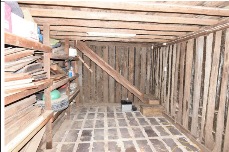
Caption: Barn at 37-39 North Street, Windsor (interior) Photographer: S. Johnson Copyright Owner: Lucas Stapleton Johnson & Partners Pty Ltd Date: May 2023
