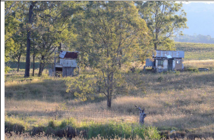
Caption: Barn at No. 33 Griffins Rd, Tennyson Photographer: G. Edds Copyright Owner: Graham Edds & Associates Date: June 2023
