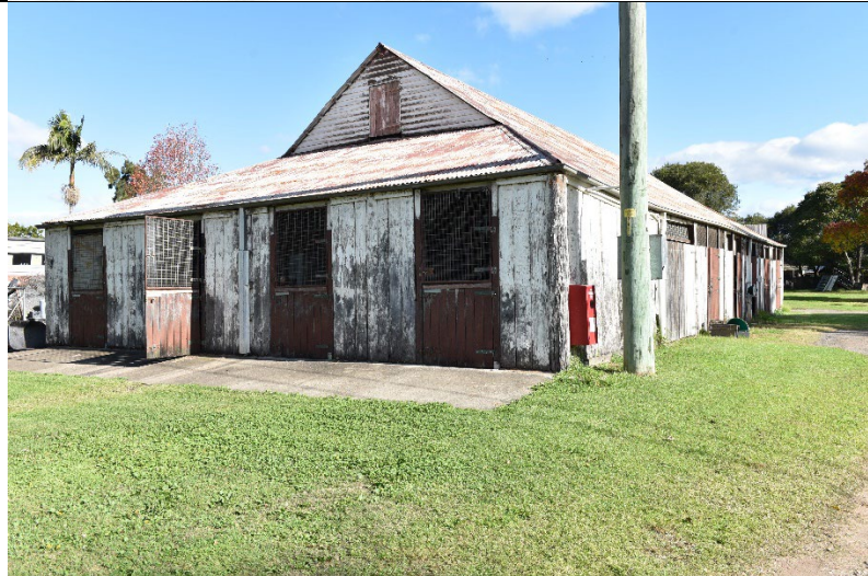
Caption: Barn 1 at 331 Hobartville, 36-40 Inalls Lane, Richmond (exterior) Photographer: S. Johnson Copyright Owner: Lucas Stapleton Johnson & Partners Pty Ltd Date: June 2023
