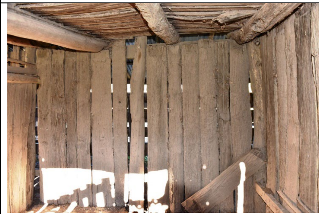
Caption: Interior detail of barn at No. 995 Upper Colo Road, Upper Colo Photographer: S. Johnson Copyright Owner: Lucas Stapleton Johnson & Partners Date: June 2023
