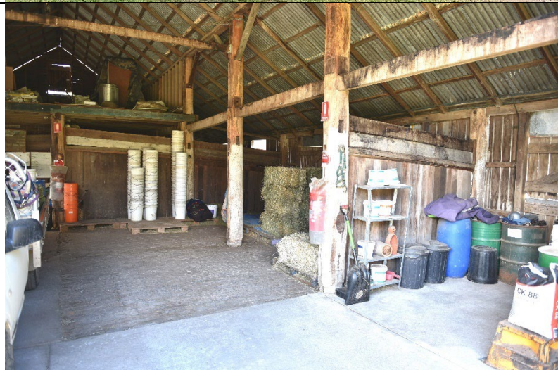
Caption: Barn 1 at 331 Hobartville, 36-40 Inalls Lane, Richmond (interior) Photographer: S. Johnson Copyright Owner: Lucas Stapleton Johnson & Partners Pty Ltd Date: June 2023
