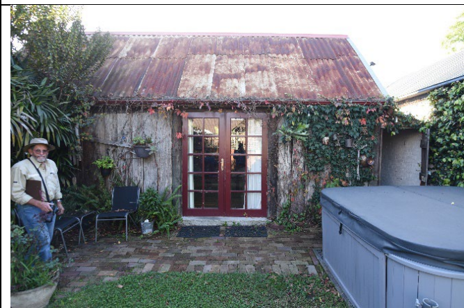
Caption: The town barn at No. 2 Catherine Street, Windsor. Photographer: K. Denny Copyright Owner: Lucas Stapleton Johnson & Partners Date: May 2023
