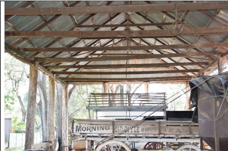
Caption: Barn 3 at 331 Hobartville, 36-40 Inalls Lane, Richmond (interior looking north) Photographer: S. Johnson Copyright Owner: Lucas Stapleton Johnson & Partners Pty Ltd Date: June 2023
