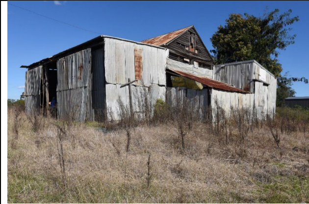
Caption: Barn at 87 Wilberforce Road, Wilberforce (exterior) Photographer: S. Johnson Copyright Owner: Lucas Stapleton Johnson & Partners Pty Ltd Date: May 2023
