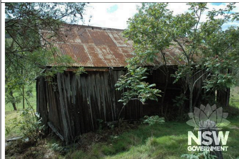
Caption: Slab barn at No. 1665 Upper Colo Road, Upper Colo. Photographer: C. Edds Copyright Owner: Graham Edds & Associates Date: 2010
