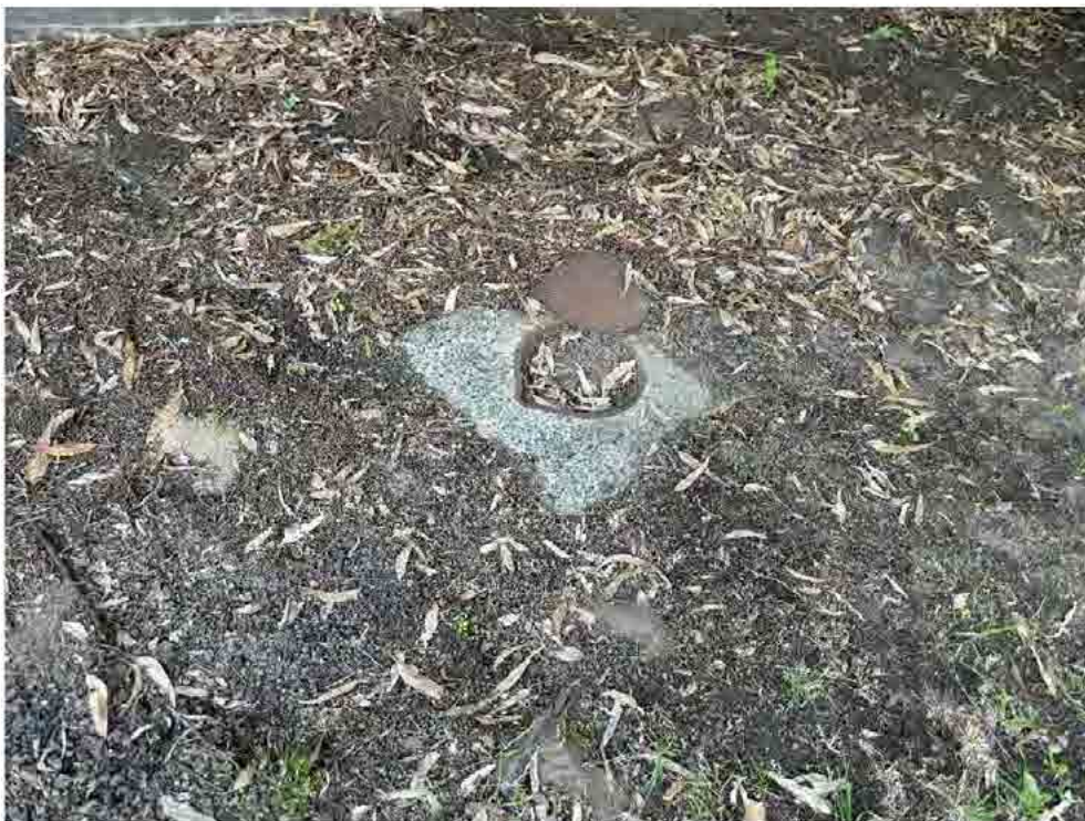
PHOTO 14 Fill / dip point in front of the fuel dispenser
