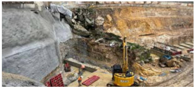
Works continued on restoring local roads, including the historic Thomas James Bridge at Lower Macdonald
