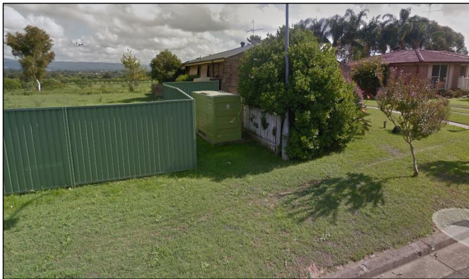
Existing Substation (S8655)
