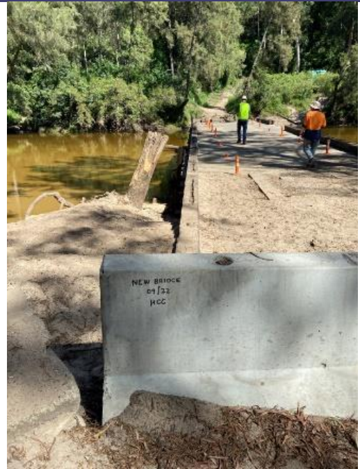
Upper Colo Bridge. Damaged by flooding in 2021
