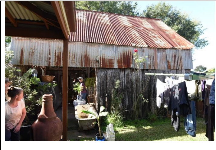
Caption: The town barn at No. 4 Catherine Street, Windsor (exterior). Photographer: S. Johnson Copyright Owner: Lucas Stapleton Johnson & Partners Date: May 2023
