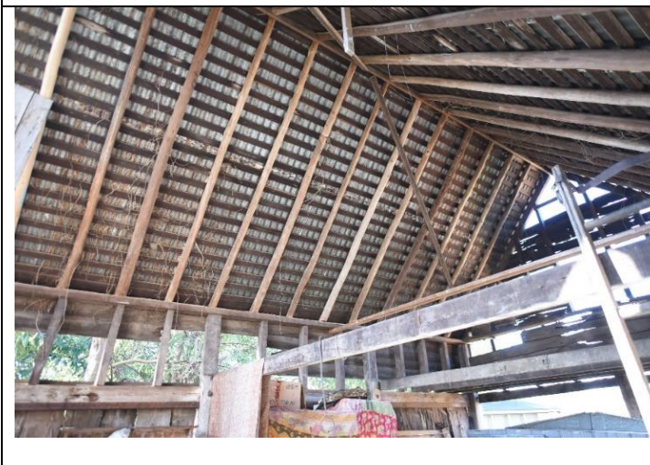
Caption: The town barn at No. 4 Catherine Street, Windsor (interior). Photographer: S. Johnson Copyright Owner: Lucas Stapleton Johnson & Partners Date: May 2023
