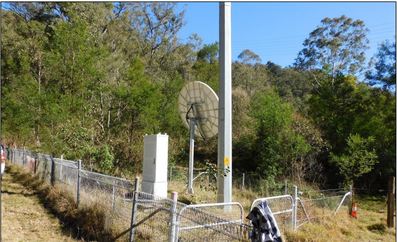
Figure 7: Photo taken during a site visit showing the location of the existing small cell facility and proposed Telstra compound within a cleared portion of land
