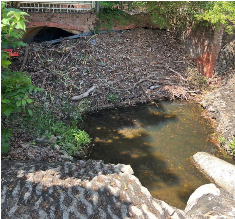
Figure 5.4 Photograph of inspected blocked culvert in the urbanised area (North Richmond)
