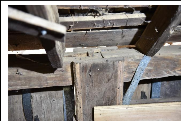
Caption: Detail of pegged joint between post and beam in barn at 164 Old Bells Line of Road, Kurrajong Photographer: S. Johnson Date: June 2023
