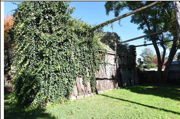
Caption: Barn 2 at No. 20-22 Buckingham Street, Pitt Town Photographer: S. Johnson Copyright Owner: Lucas Stapleton Johnson & Partners Date: May 2023
