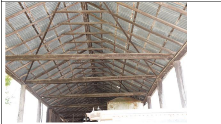
Caption: Roof structure of barn at 176B Hibberts Lane, Freemans Reach Photographer: S. Johnson Date: June 2023
