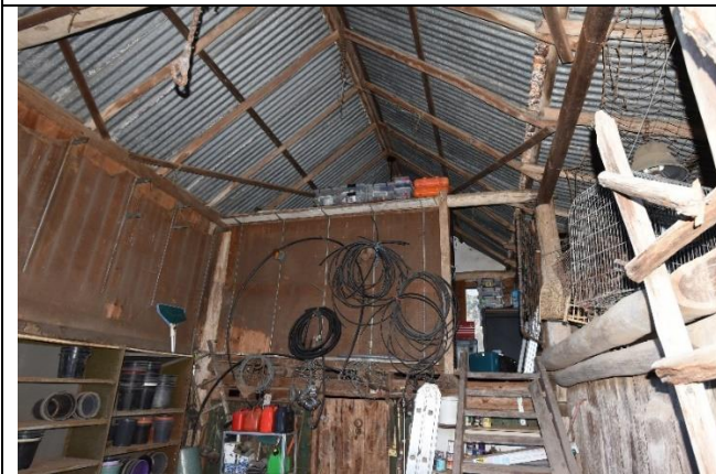
Caption: Barn at 30 Wolseley Road, McGraths Hill (interior) Photographer: K. Denny Copyright Owner: Lucas Stapleton Johnson & Partners Pty Ltd Date: May 2023
