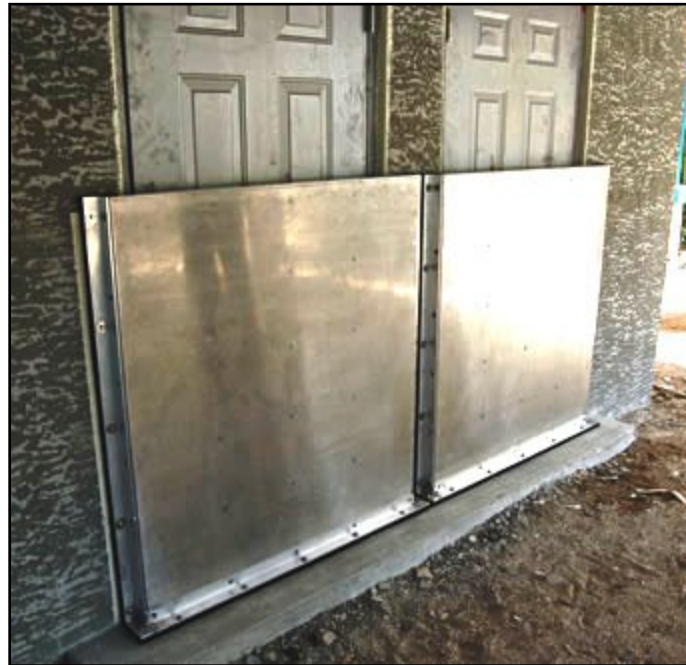
Photo 2: Dry proofing on doors of residential property
