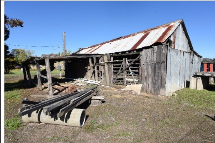
Caption: Former blacksmith workshop and house at No. 292 Pitt Town Road, Pitt Town (exterior) Photographer: S. Johnson Copyright Owner: Lucas Stapleton Johnson & Partners Date: May 2023
