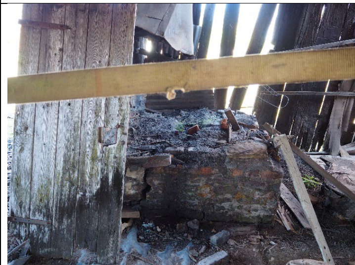
Caption: Brick hearth inside former blacksmith workshop at No. 292 Pitt Town Road, Pitt Town Photographer: S. Johnson Copyright Owner: Lucas Stapleton Johnson & Partners Date: May 2023
