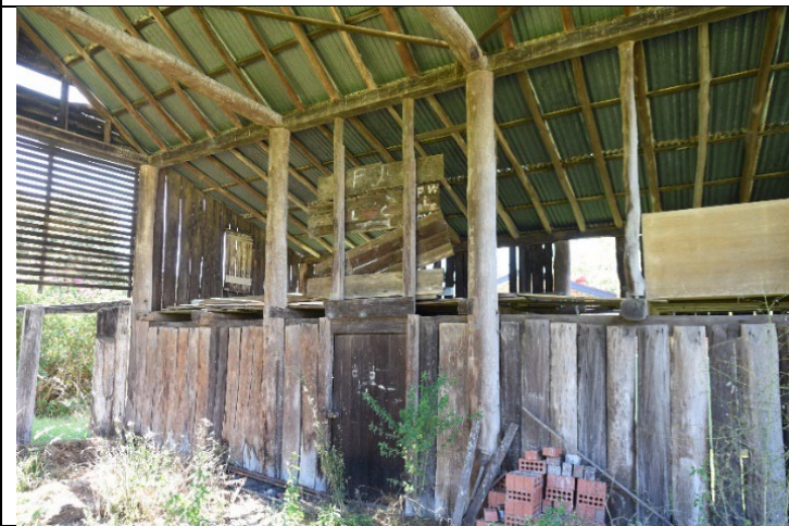
Caption: Barn at No. 26A Buckingham Street, Pitt Town (interior view) Photographer: S. Johnson Copyright Owner: Lucas Stapleton Johnson & Partners Date: May 2023
