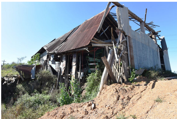
Figure 6. 3: Early 19 th century slab barn at No. 56 Freemans Reach Road, Freemans Reach showing the impacts of 2022 floods on the structure as a result of the washing away of river bank.
