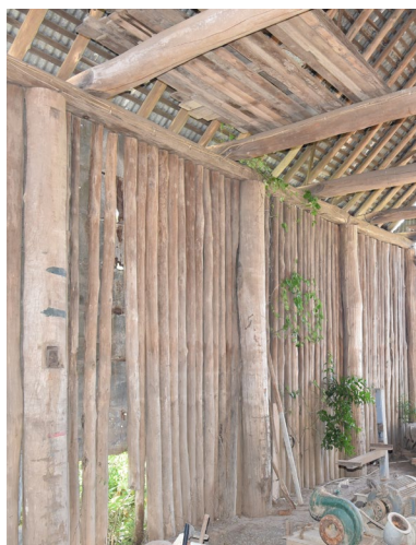
Figure 3. 28: Detail of palisade wall cladding and shingle battens to barn at No 56 Freemans Reach Road, Freemans Reach.
