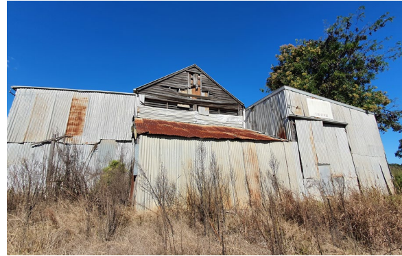
Figure 3. 32: Weatherboard infill to gable end of main barn at No. 87 Wilberforce Road including loft door.
