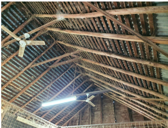
Figure 3. 26: Barn 2 'Bottom stables' at Hobartville, No.36-40 Inalls Lane, Richmond with pole rafters and shingle battens.
