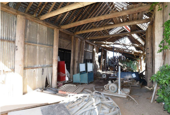
Figure 3. 15: Interior of main body of single storey barn at No. 56 Freemans Reach Road, Freemans Reach showing roof structure.
