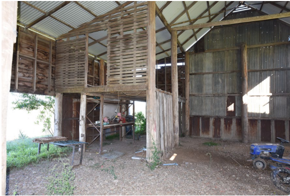
Figure 3. 17: Loft structure in skillion addition in barn at No. 353 Freemans Reach Road, Freemans Reach.
