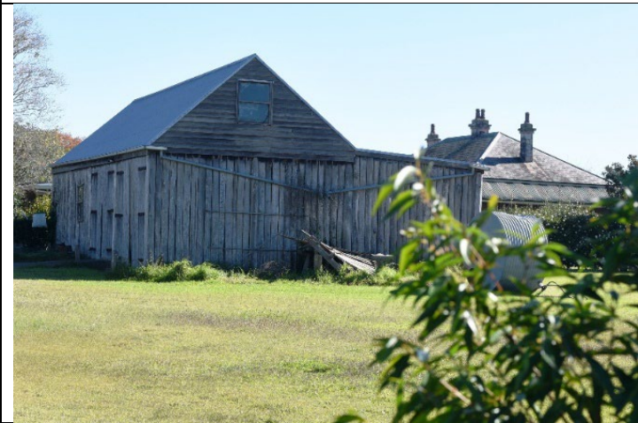
Caption: Barn E at Bona Vista complex Photographer: S. Johnson Copyright Owner: Lucas Stapleton Johnson & Partners Date: May 2023
