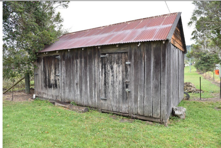
Caption: Shed at 5 Bowen Mountain Road, Grose Vale (exterior) Photographer: S. Johnson Copyright Owner: Lucas Stapleton Johnson & Partners Pty Ltd Date: June 2023
