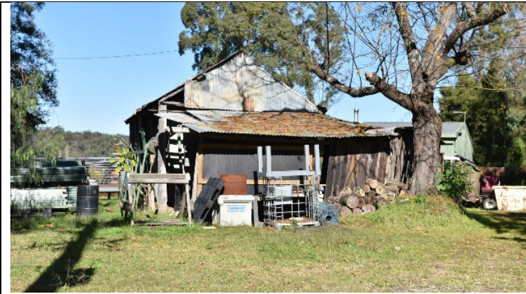
Caption: Barn at 1280 West Portland Road, Lower Portland Photographer: S. Johnson Copyright Owner: Lucas Stapleton Johnson & Partners Date: June 2023
