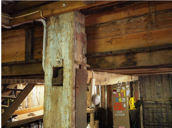
Caption: Through tenon joint between cross beam and post in barn at 164 Old Bells Line of Road, Kurrajong Photographer: S. Johnson Date: June 2023
