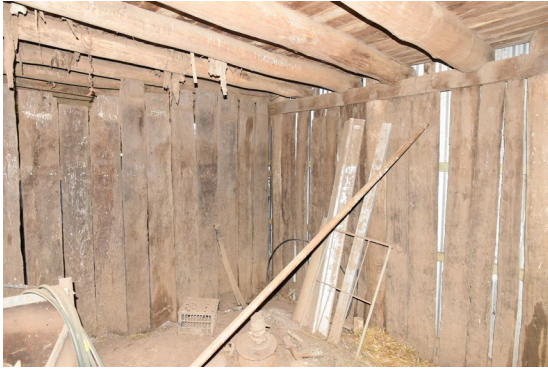
Figure 3. 31: Internal view of barn at No. 331 Freemans Reach Road, Freemans Reach with slab wall cladding and corrugated iron over externally.
