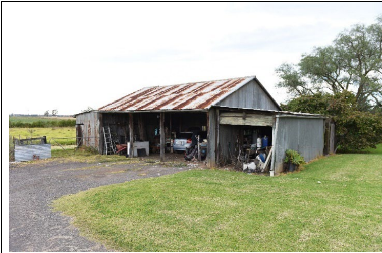
Caption: Barn at 121 Blacktown Road, Freemans Reach (exterior) Photographer: K. Denny Copyright Owner: Lucas Stapleton Johnson & Partners Date: June 2023
