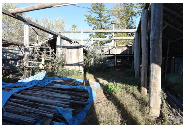
Figure 6. 10: View of interior of Tebbutt’s Barn in May 2023 showing salvaged and stored building components waiting reconstruction works.
