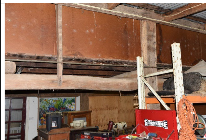
Caption: View from skillion of Barn 1 structure, note stripes from horizontal battens Photographer: S Johnson Copyright Owner: Lucas Stapleton Johnson & Partners Date: June 2023
