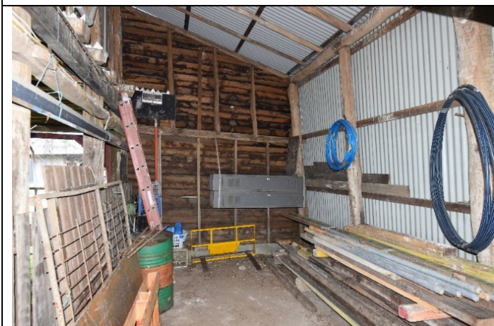
Caption: Barn at 331 Cattai Road, Cattai (interior) Photographer: S. Johnson Copyright Owner: Lucas Stapleton Johnson & Partners Pty Ltd Date: May 2023
