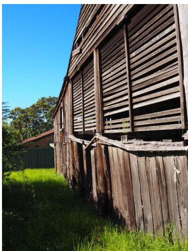
Figure 3. 29: Detail of timber vertical slabs and horizontal slats to barn at No. 26A Buckingham Street, Pitt Town.
