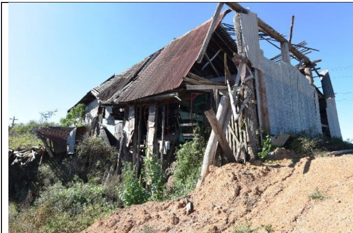
Caption: Barn at 56 Freemans Reach Road, Freemans Reach (exterior) Photographer: S. Johnson Copyright Owner: Lucas Stapleton Johnson & Partners Pty Ltd Date: May 2023
