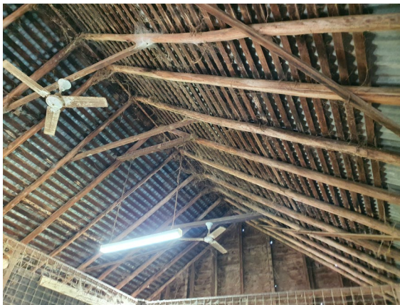
Figure 3. 26: Barn 2 'Bottom stables' at Hobartville, No.36-40 Inalls Lane, Richmond with pole rafters and shingle battens.
