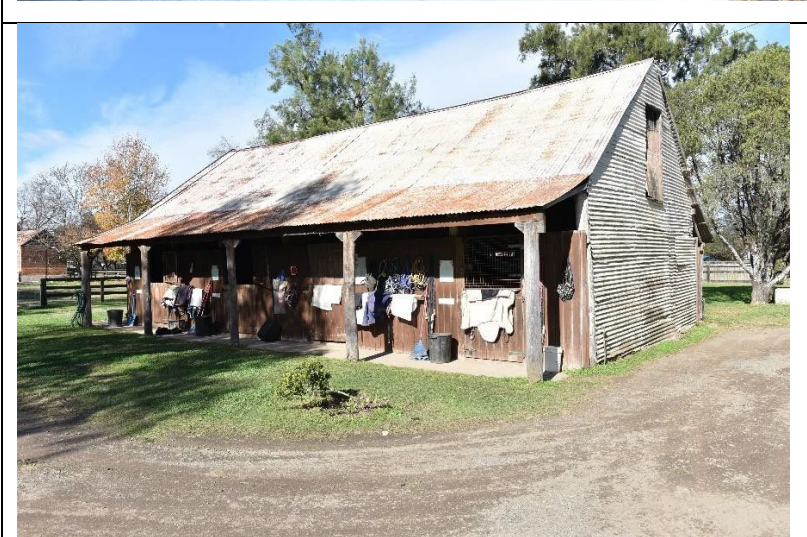
Caption: Barn 2 at 331 Hobartville, 36-40 Inalls Lane, Richmond (exterior) Photographer: S. Johnson Copyright Owner: Lucas Stapleton Johnson & Partners Pty Ltd Date: June 2023
