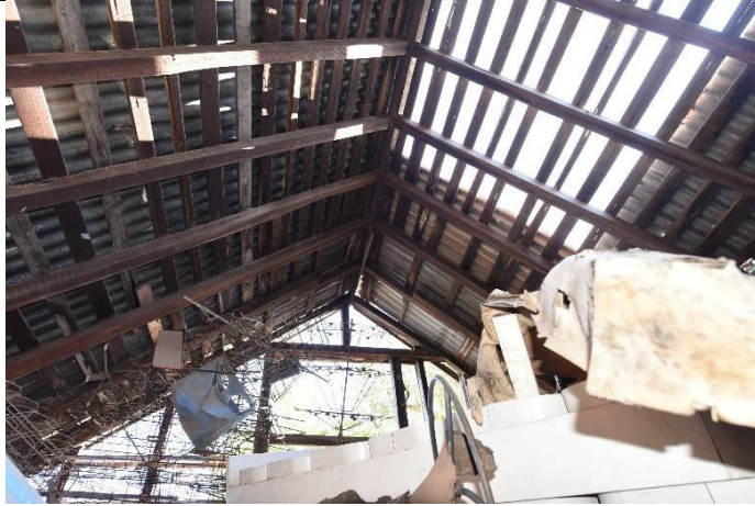
Caption: Town barn at 117 George Street, Windsor (detail) Photographer: S. Johnson Copyright Owner: Lucas Stapleton Johnson & Partners Pty Ltd Date: May 2023
