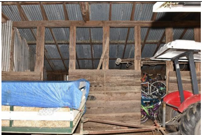
Caption: Detail of posts and beam separating main barn from skillion (note evidence of loft support), No. 496 Wilberforce Road, Wilberforce Photographer: S. Johnson Copyright Owner: Lucas Stapleton Johnson & Partners Date: July 2023
