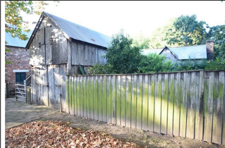
Caption: Barn at 37 -39 North Street, Windsor (exterior) Photographer: S. Johnson Copyright Owner: Lucas Stapleton Johnson & Partners Pty Ltd Date: May 2023
