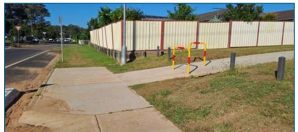
Barriers on new path from Stewart St heading towards Batten Circuit – slight incline.
