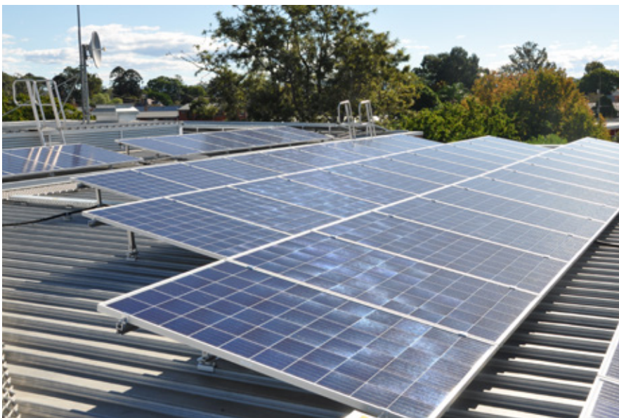
Figure 4: Solar panels in the Hawkesbury City Council Administration Precinct
