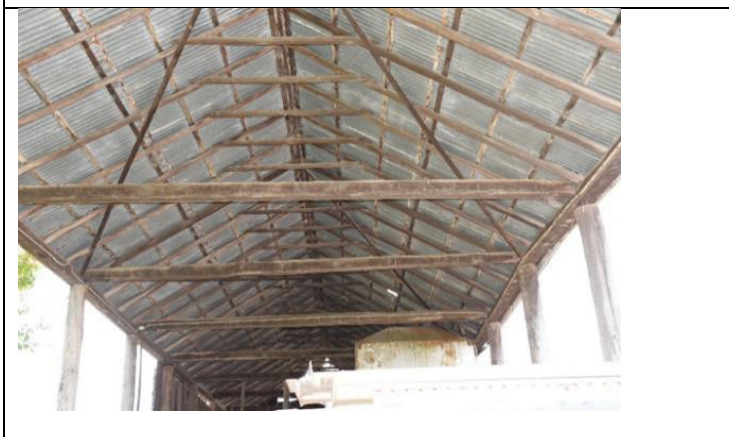
Caption: Roof structure of barn at 176B Hibberts Lane, Freemans Reach Photographer: S. Johnson Date: June 2023
