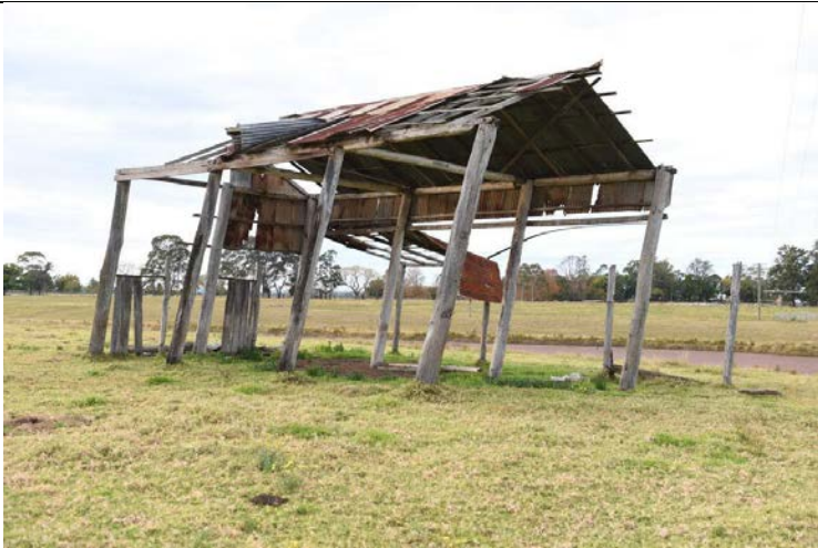
Caption: Barn at 37-97 Gorricks Lane, Freemans Reach (exterior) Photographer: S. Johnson Copyright Owner: Lucas Stapleton Johnson & Partners Pty Ltd Date: June 2023
