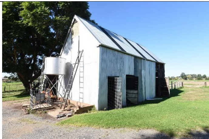
Caption: Barn A at 331 Freemans Reach Road, Freemans Reach (exterior) Photographer: LSJ Copyright Owner: Lucas Stapleton Johnson & Partners Pty Ltd Date: May 2023
