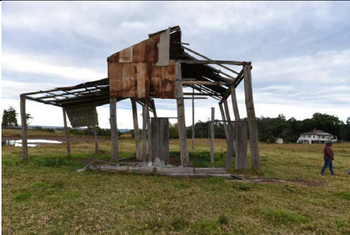
Caption: Barn at 37-97 Gorricks Lane, Freemans Reach (exterior) Photographer: S. Johnson Copyright Owner: Lucas Stapleton Johnson & Partners Pty Ltd Date: June 2023
