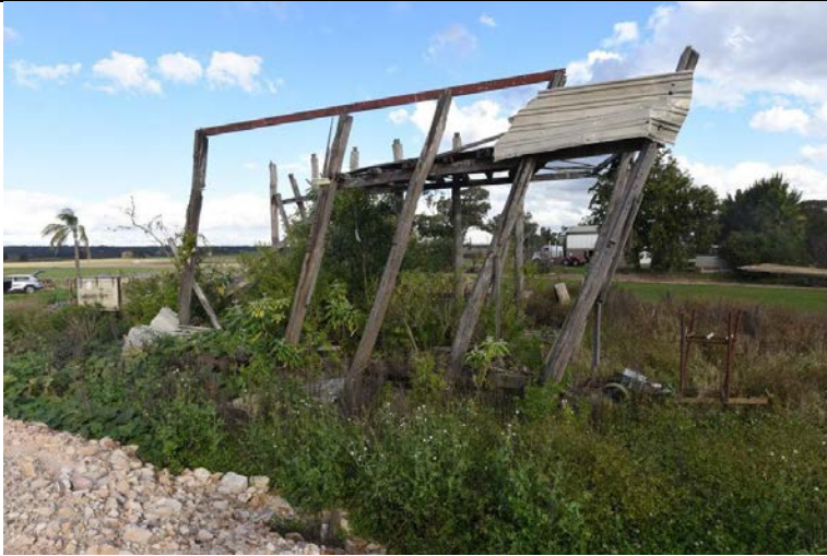
Caption: Barn at 283 Pitt Town Bottoms Road, Pitt Town Bottoms (exterior) Photographer: LSJ Copyright Owner: Lucas Stapleton Johnson & Partners Pty Ltd Date: May 2023:
