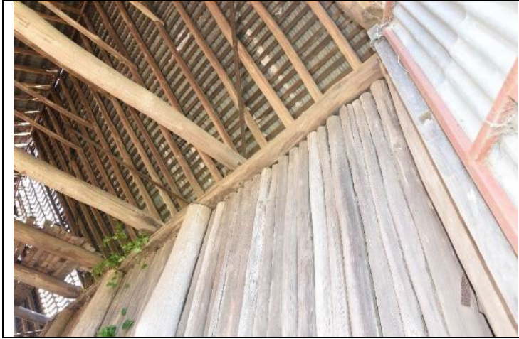
Caption: Barn at 56 Freemans Reach Road, Freemans Reach (interior) Photographer: S. Johnson Copyright Owner: Lucas Stapleton Johnson & Partners Pty Ltd Date: May 2023
