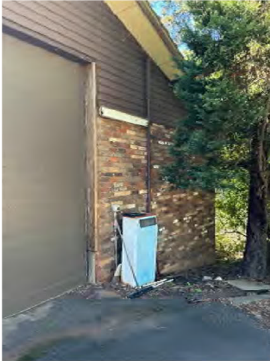
PHOTO 13 Observed fuel dispenser and vent for the UST
