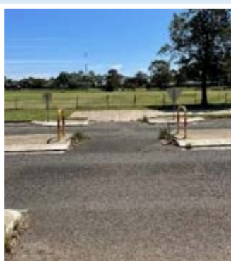
Figure 25: Pedestrian refuge island on Berger Road, South Windsor
